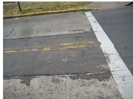
Poor pavement quality, such as on this stretch of University Street, can be a hazard for bicyclists.
