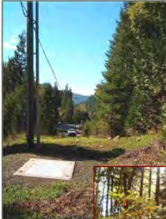
Top: Connection from overhead power to vault.
