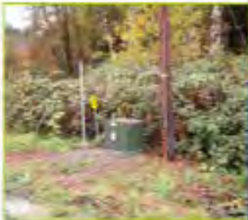
Top: Abandoned above ground line easement showing susceptibility to falling vegetation damages.
